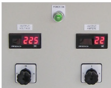
Digital Output Voltmeter & Ammeter with phase selector switches
