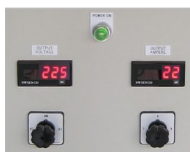
Digital Output Voltmeter & Ammeter with phase selector switches
