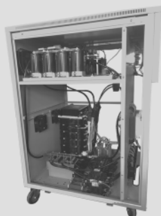
Typical Internal View - 45 kVA Model
